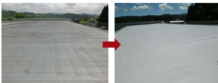
Energy saving by application of water-proof anti-heat paint on roof (Engineering & development center)
