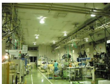
Mold building: Replaced mercury lamps with ceramic metal light and light thinning for energy saving.
