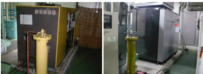
Miyazaki Fujitsu Components Limited Replaced 75kw compressors with energy-saving ones and applied sound deadening treatment
