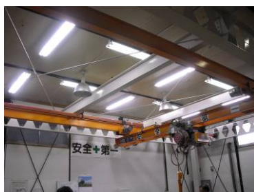
Press building: Replaced mercury lamps with Hf fluorescent and turned off remained mercury lamps for energy saving.
