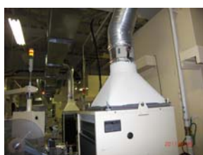
Heat insulating coat on exhaust heat duct
