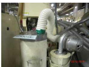
Exhaust heat to outdoor Shinano Fujitsu Limited
