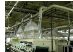
Reduction of air-cooling load by forced exhaust system Shinano Fujitsu Limited
